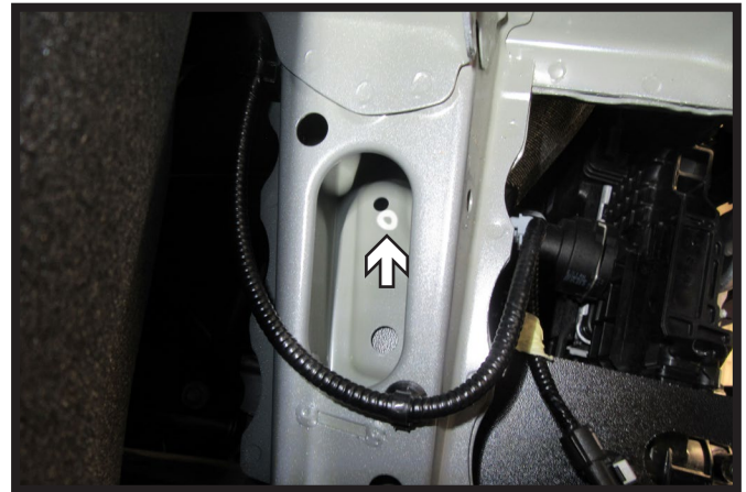
15. Hold the support plate in place on passenger side of the vehicle so the front holes and back bottom hole line up with the existing holes on the vehicle. Mark frame using the baseplate as a template for top back hole.
